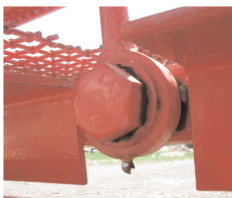
Inspect all Dog Bones every day for cracks or damage.
