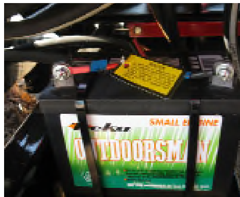
Battery — check connections/disconnect before working on electric system
