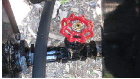
Hydraulic oil tank shut off valve
